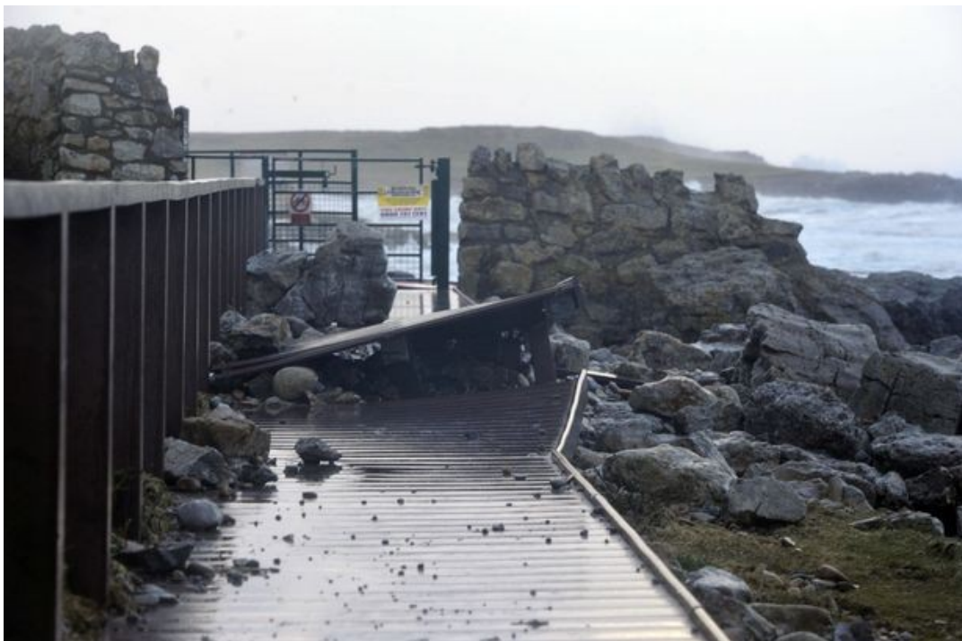
Damage on the Ceredigion Coastal Path caused by winter storms.
